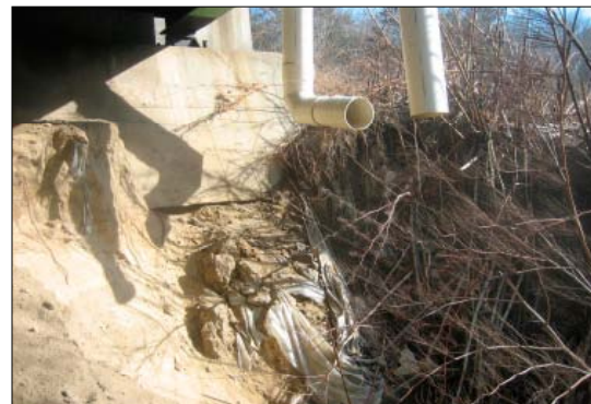
EROSION AT MOUSAM RIVER BRIDGE
