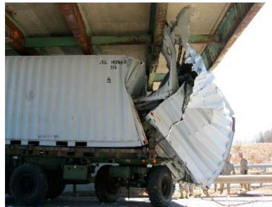
INTERCHANGE 102 UNDERPASS HIGH LOAD HIT
