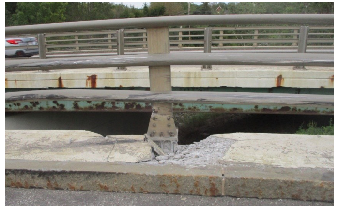
CENTRAL STREET OVERPASS BRIDGE RAIL DAMAGE
